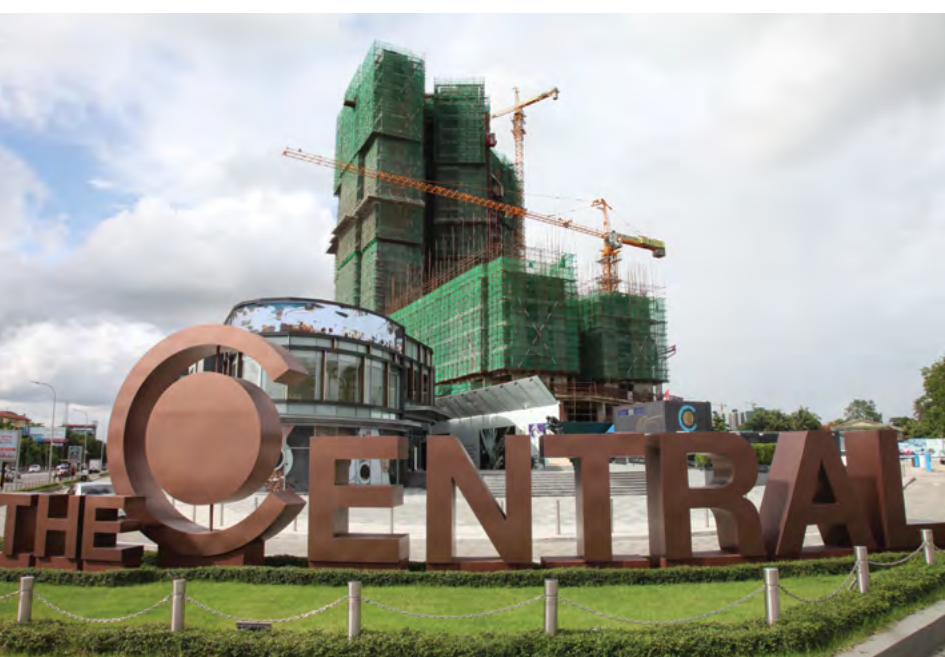
Marga Landmark has selected Cummins QSK60 gensets for phase one of 'The Central' – a flagship project in downtown Yangon.
