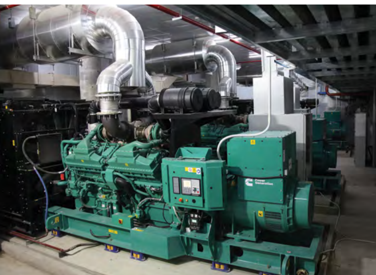
Three 2250 kVA gensets come on line within 10 seconds when signalled by the Cummins PowerCommand on-board control system.
