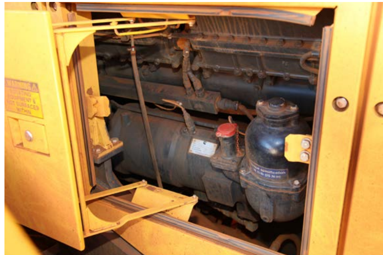
Eliminator oil filtration system is a natural fit in the WA1200 engine bay.
