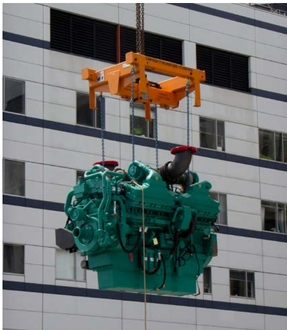
Cummins QSK60 on its way to the plant room on the hospital roof.
