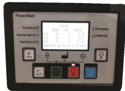
PowerStart 600 control operator /display panel
